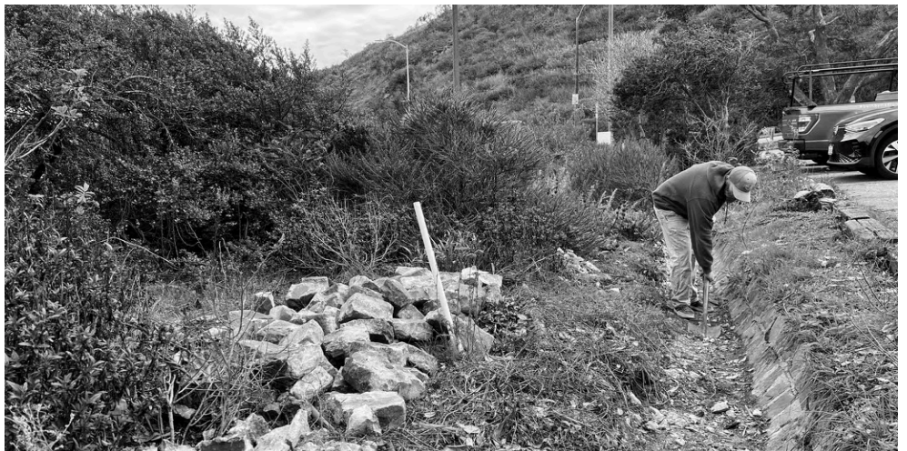
Removing the cobblestones in the trench for future use in the crushed rock path and patio
